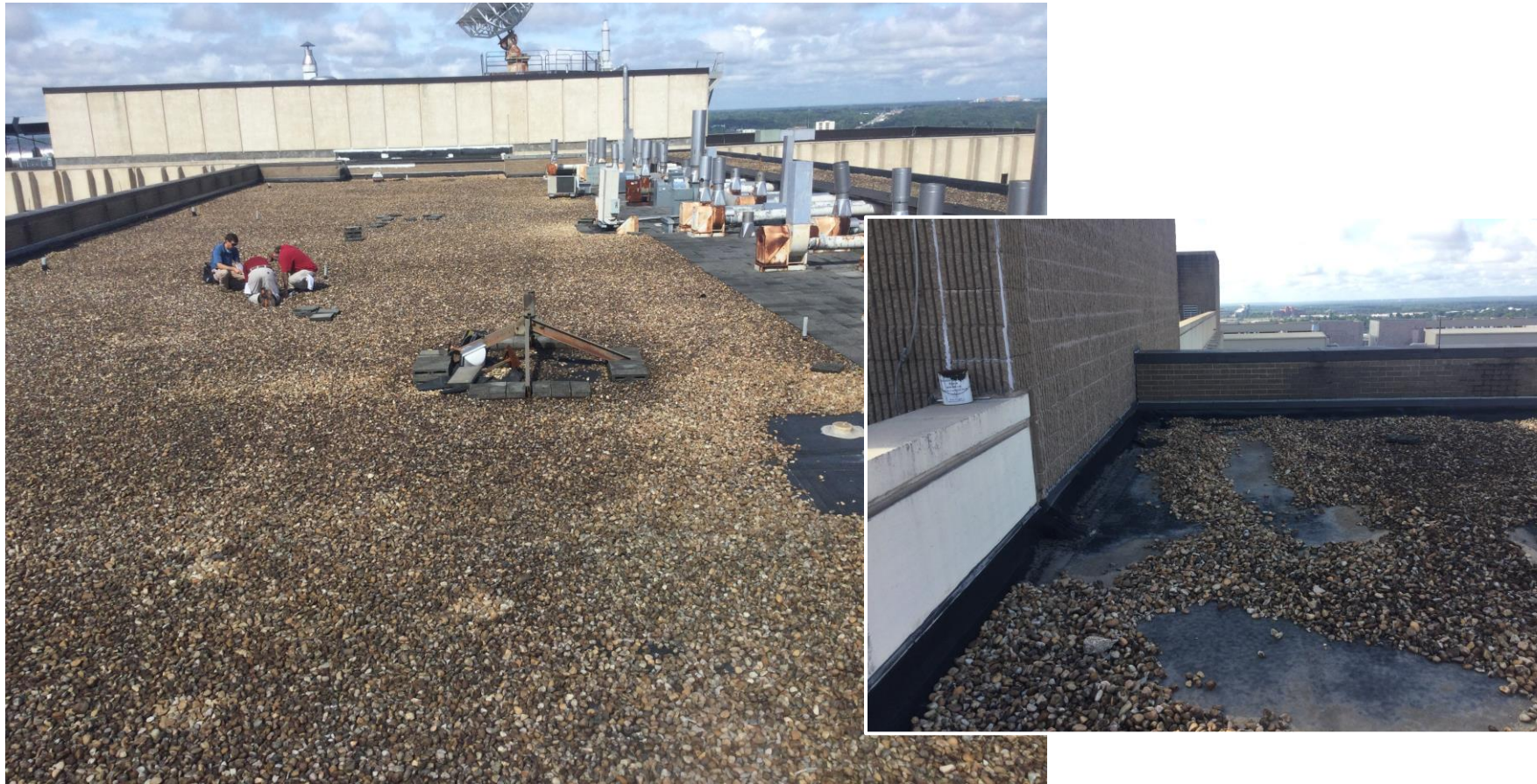
Deteriorated roof membrane and ballast
